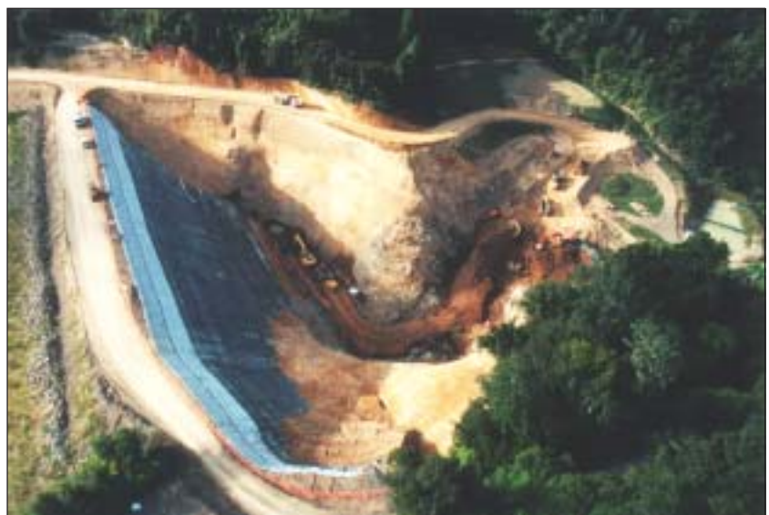
Figure 3. Cosseys Dam with the face removed to allow the installation of the underdrain and filter.
