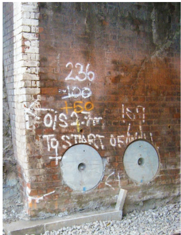
Rock anchors near a tunnel portal. Image courtesy of Kevin Jones Archaeologist Ltd.
