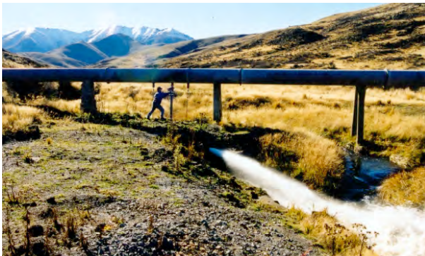
Figure 7. Wetherburn syphon sluice valve in operation
