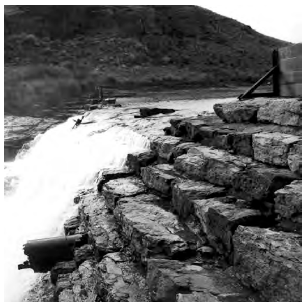
Figure 18. Lake Onslow Dam 1968 flood damage and showing masonry construction
