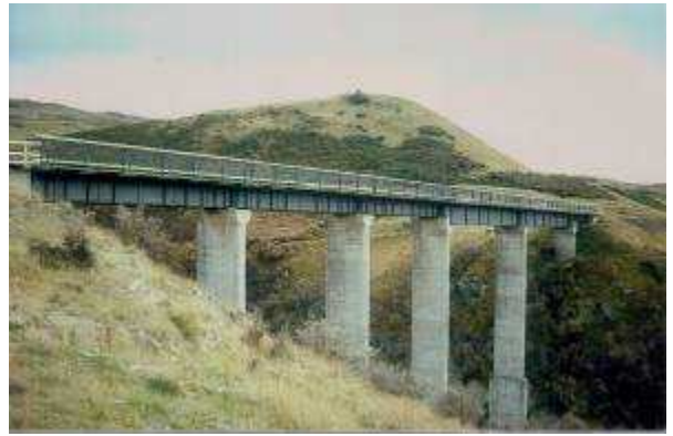
Figure 13. Prices Creek viaduct near Hyde, built in early 1960's it was the last bridge built on the line.
