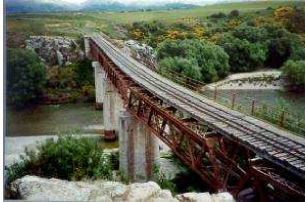
Figure 11. Manuherikia No. 1 bridge was the first built using concrete for the piers.
