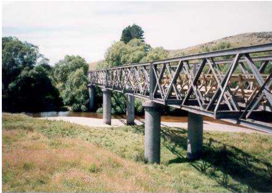
Figure 2. The bridge over the Taieri River near Waipiata illustrates one of the many engineering styles used on the Otago Central branch line.
