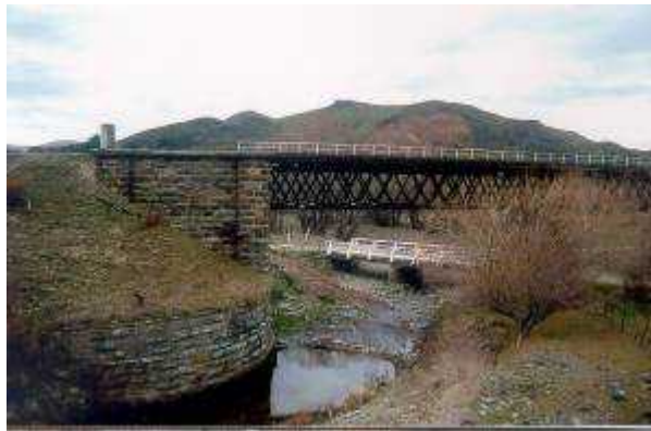
Figure 8. The Capburn Bridge at Tiroiti showing fine stone work abutments and lattice sub structure.
