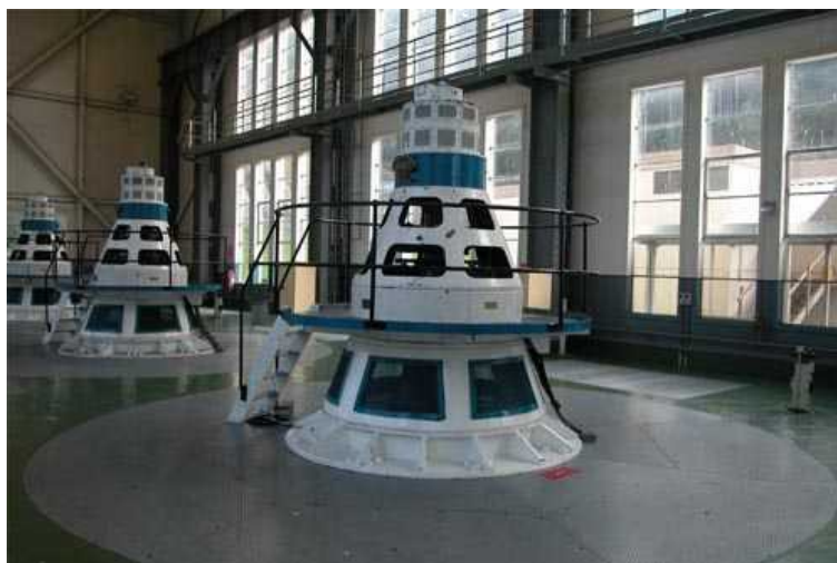
Figure 4. Tungatinah Power Station, the turbine has been rebuilt within the existing chamber and casing, retaining the appearance but not the fabric.
