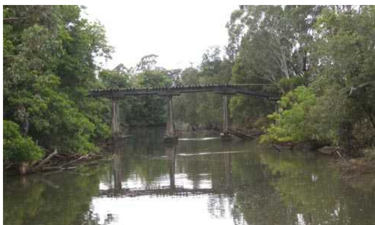
Figure 5. Bomaderry Railway Bridge, built but never used and now collapsing.
